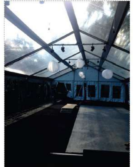
Everything leveled to perfection. Laying down the Carpet and putting on the finishing touches
