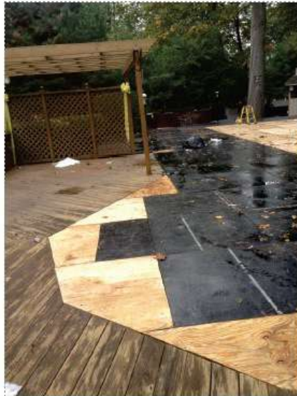
...But not for Party Line! We cut plywood and I Beams to meet the Deck and Bi-Jax evenly.
