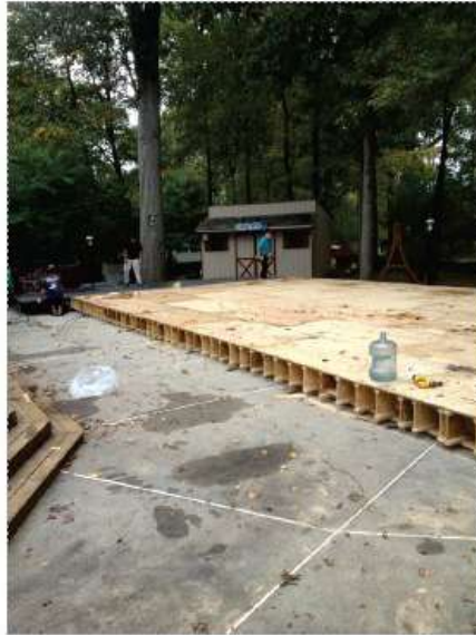
Wooden I Beams are secured to a layer of plywood for the highest level of stability over the pool area
